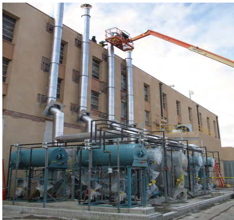
“Steam Plant Temporary Boiler Installation, SNL/NM” 2008 Photo Contest, photo by Kelsey Curran
